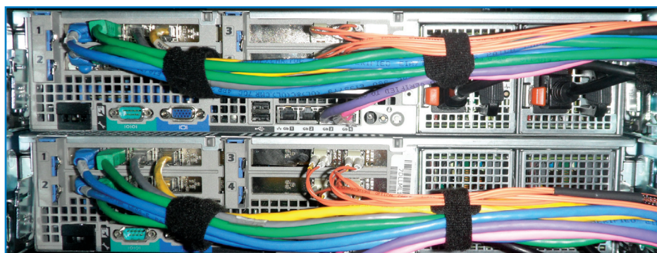
Figure 1. Multiple gigabit Ethernet connections in a typical virtualized server.
